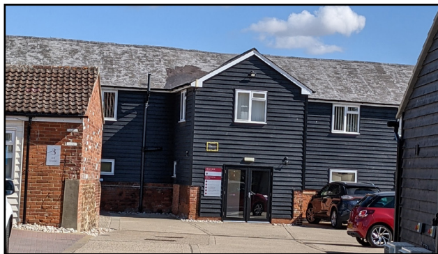
Figure 23 Loss of historic features within the barn complex can be seen with replacement windows, doors and roofing
