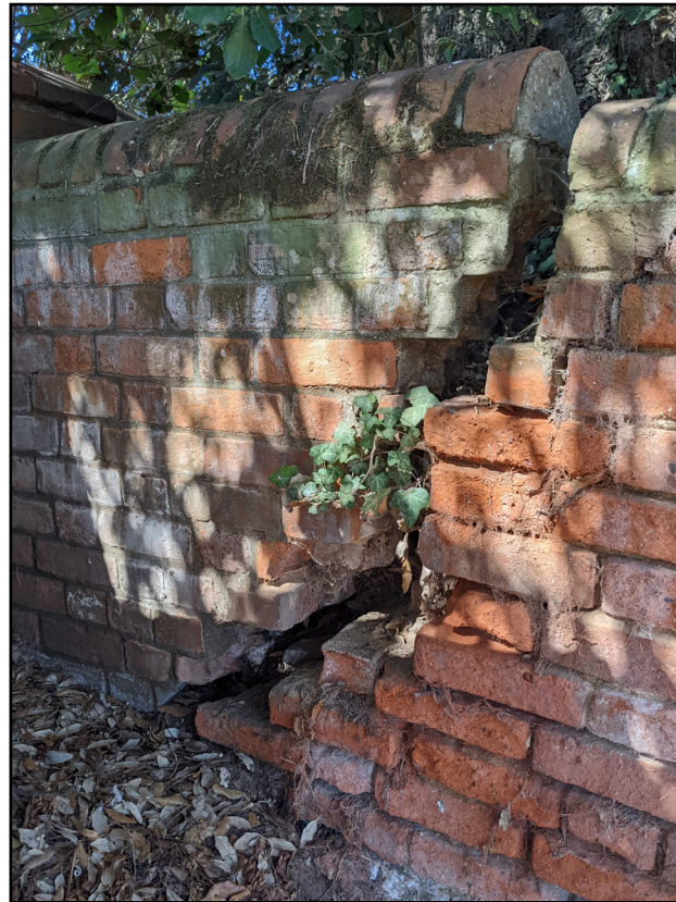
Figure 24 Damage to Brightlingsea Hall boundary wall
